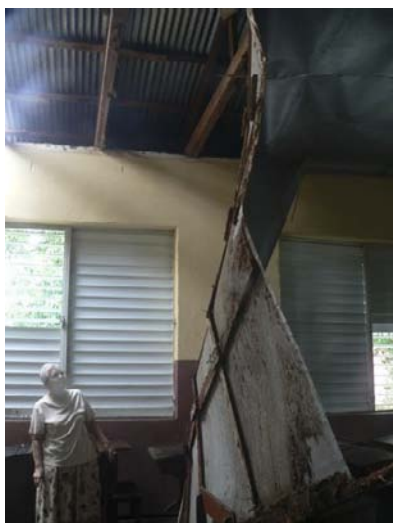
Tremendous damage caused by the hurricanes
